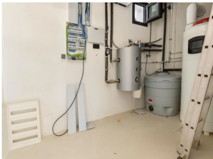
Technical room of the energy-efficient villa
