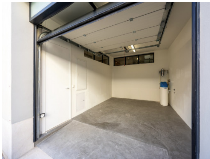
Garage with e-charging station
